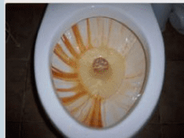
Hard water stains
